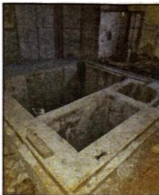
Scenes from the interior of the new mikvah under construction in Maplewood.
