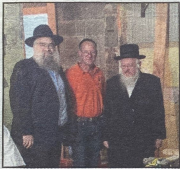
Rabbi Sholom Bogomilsky, spiritual leader of MJC (left), with project manager Jonathan Friedman and the inspecting rabbi from Mikvah USA as the foundation is formed for the first kosher mikvah in Maplewood.
